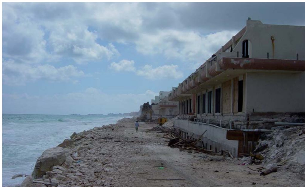
Figure 3: Beach erosion and wave damage. Source: Authors.
